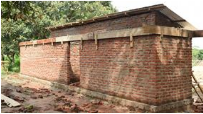
Photo 13. Ongoing construction of toilet for village dispensary (up to roofing stage) at Chabima village in Kilosa
