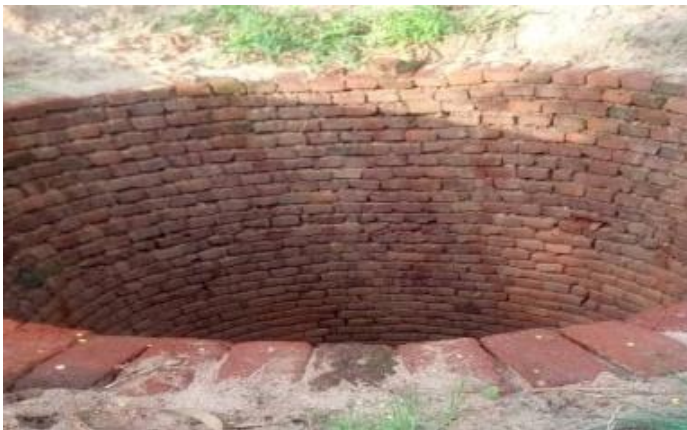
Photo 11. Ongoing construction of pit latrine for primary school at Ulaya Mbuyuni in Kilosa
