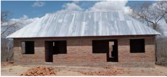
Photo 7. Ongoing construction of teachers' house (two in one) for Mlilingwa village primary in Morogoro.
